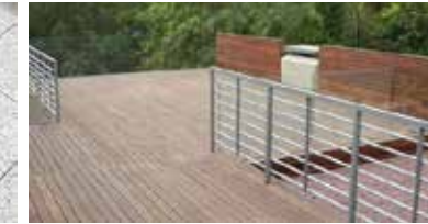
2 Wood Decking on Pedestal System
